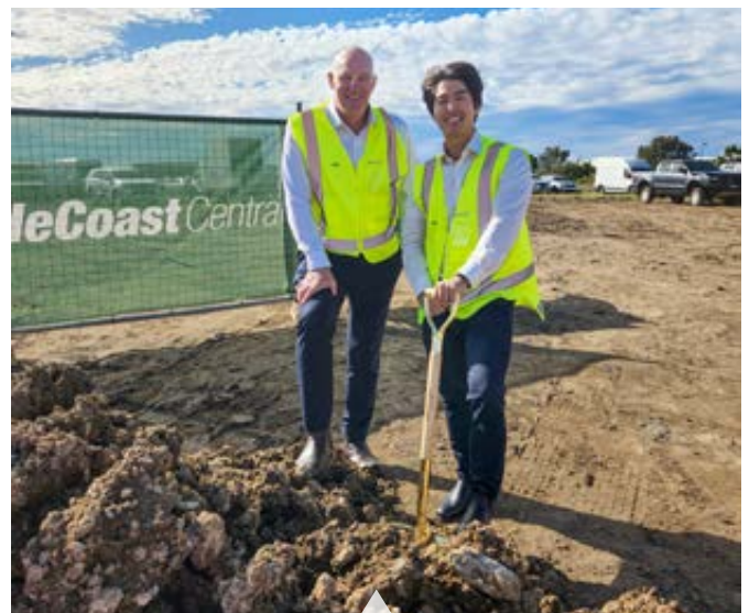
Mainfreight Team members Grant Draper and Steven Hong breaking the ground on site
